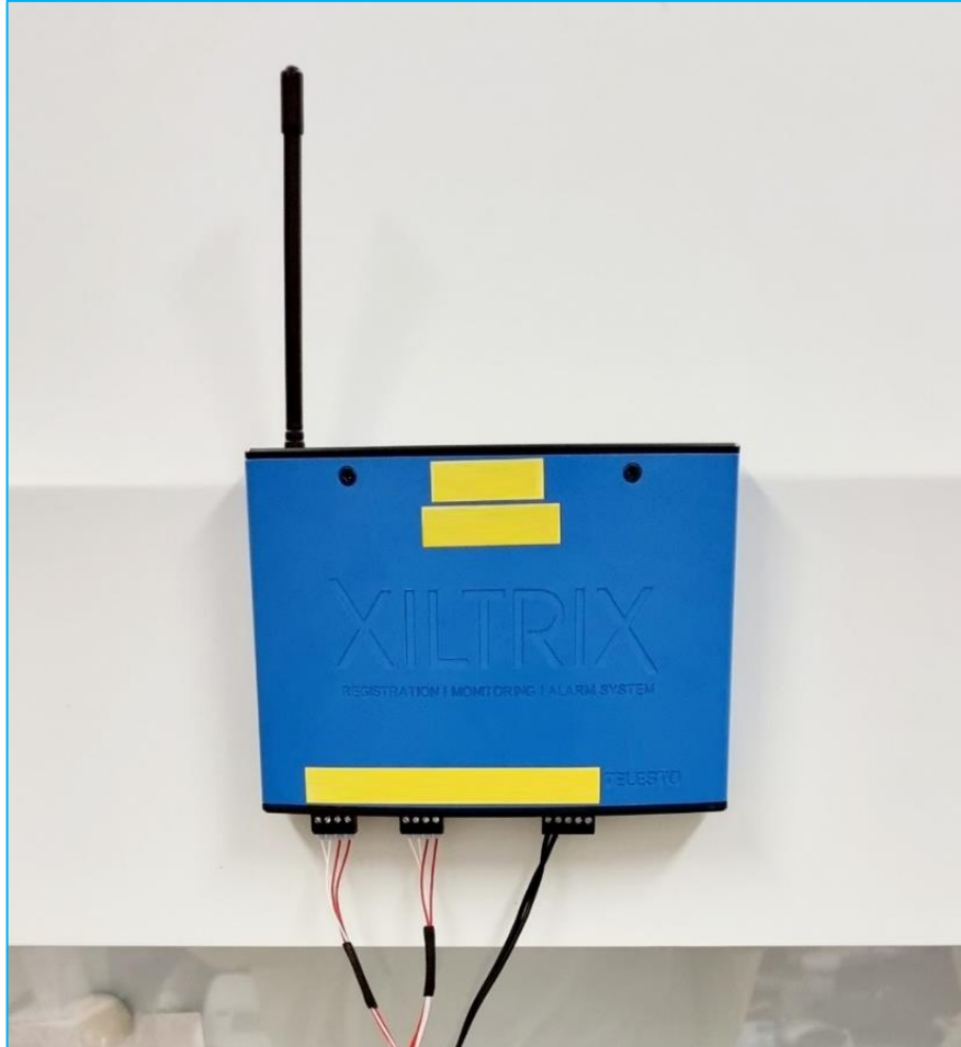
Figure 5: Example of wireless monitoring substation used for surface temperature sensors.
